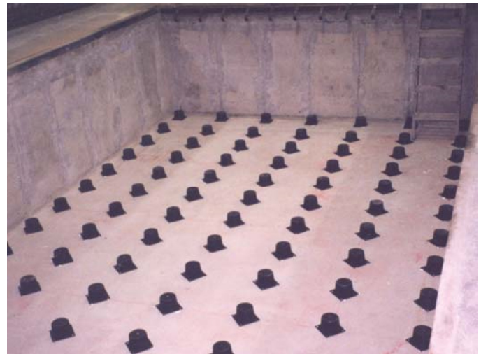
Type 2T Infab™ isolators positioned on pit floor prior to forming the foundation above.
