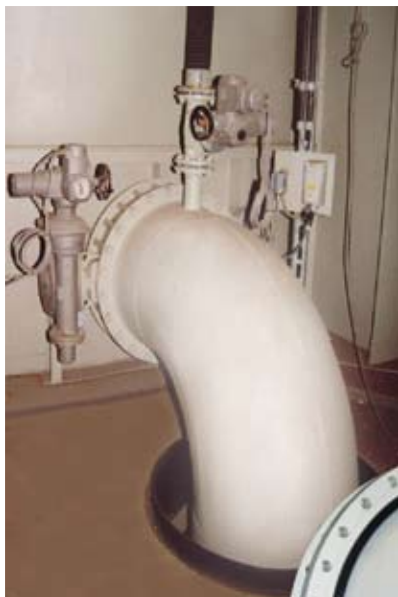
The clean installation of Center Line® RS valves.
